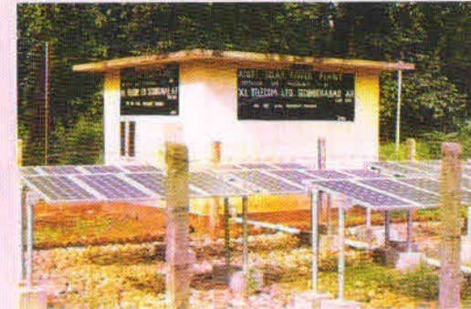
Solar Photovoltaic Power Plant (3.08 kWp) at Mundakkadavu, Malappuram Dt.
