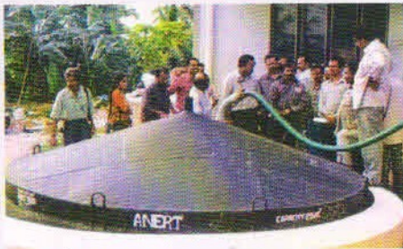
A 25m 3 Institutional Bio- gas Plant based on canteen waste installed at Hindustan Latex, Thiruvananthapuram
