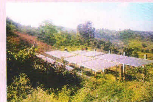
A view of the Solar Array of SPV Power Plant (3.36kWp) at Vellakulam, Palakkad Dt.
